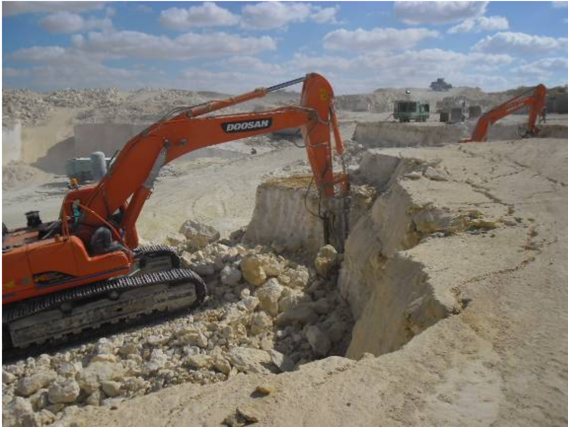
Activities at Crusher and marble area in North side of the area 28 29 57.1 N 30 15 8.4
