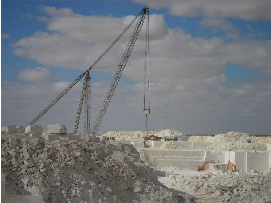
Activities at Crusher and marble area in North side of the area 28 29 57.1 N 30 15 8.4
