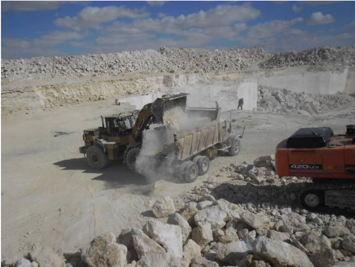
Activities at Crusher and marble area in North side of the area 28 29 57.1 N 30 15 8.4
